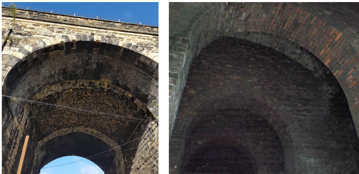
Insert 2-5 Evidence of widening of the viaduct in the 1880s, visible in the masonry; straight joints showing widened arches (left) and internal relieving arches (right).
