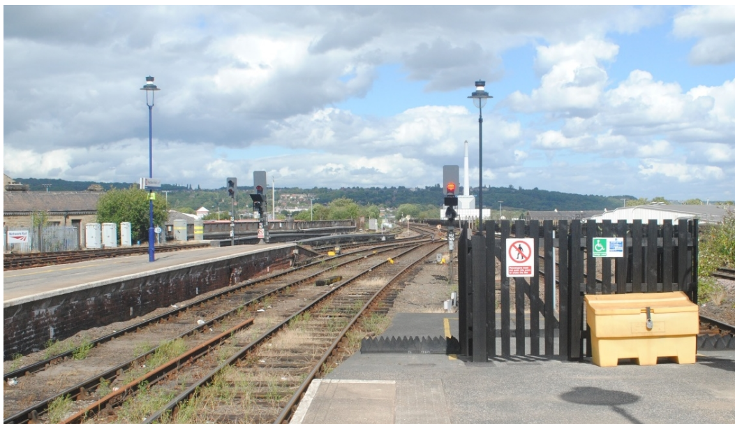
Insert 2-6 View north from the northern end of Huddersfield Station platforms along the deck of Huddersfield Viaduct (MVL3/92).
