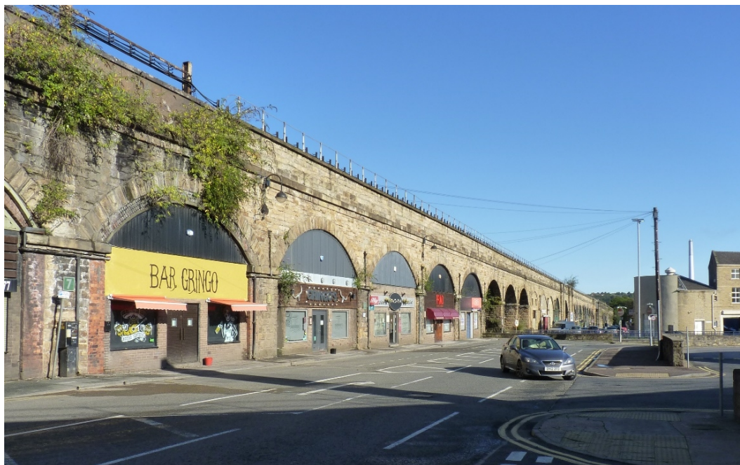
Insert 2-1 Eastern elevation of Huddersfield Viaduct (MVL3/92), viewed from southern end of Viaduct Street.
