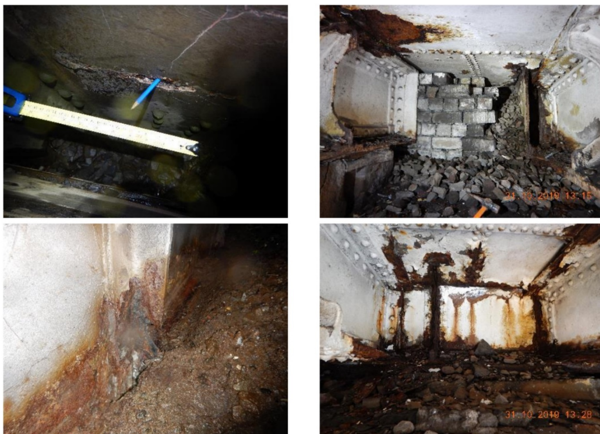
Insert 1-3 Detail of metallic spans over Northgate / Bradford Road (Span 29), showing evidence of corrosion to web and stiffeners (left) and to the members close to the I-girder connection (right).
