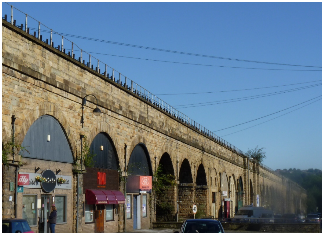
Insert 1-1 Eastern elevation of Huddersfield Viaduct (MVL3/92), looking north along Viaduct Street.
