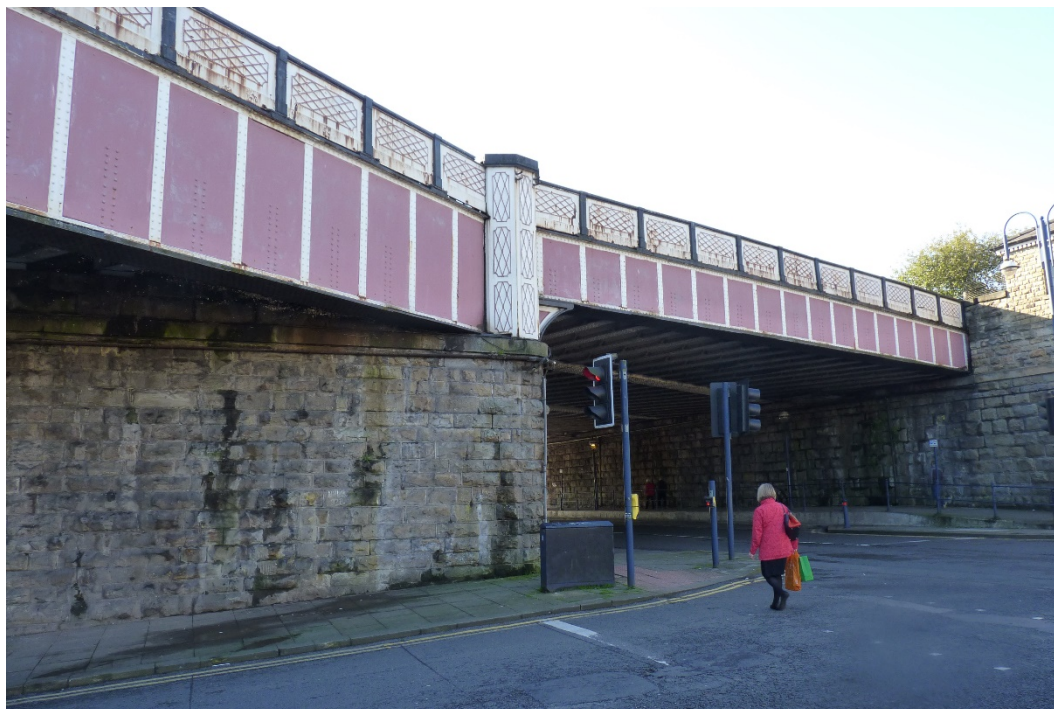
Insert 2-2 Western elevation of Huddersfield Viaduct (MVL3/92) , showing metallic spans of Fitzwilliam Street (Span 4) (left) and John William Street (Span 1) (right).
