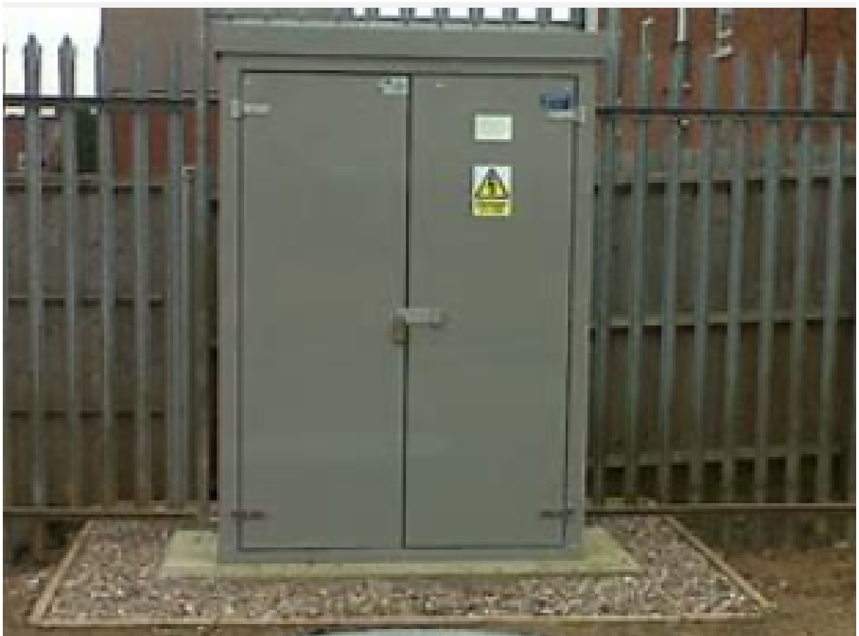
Insert 2-10 Example DNO kiosk equipment
