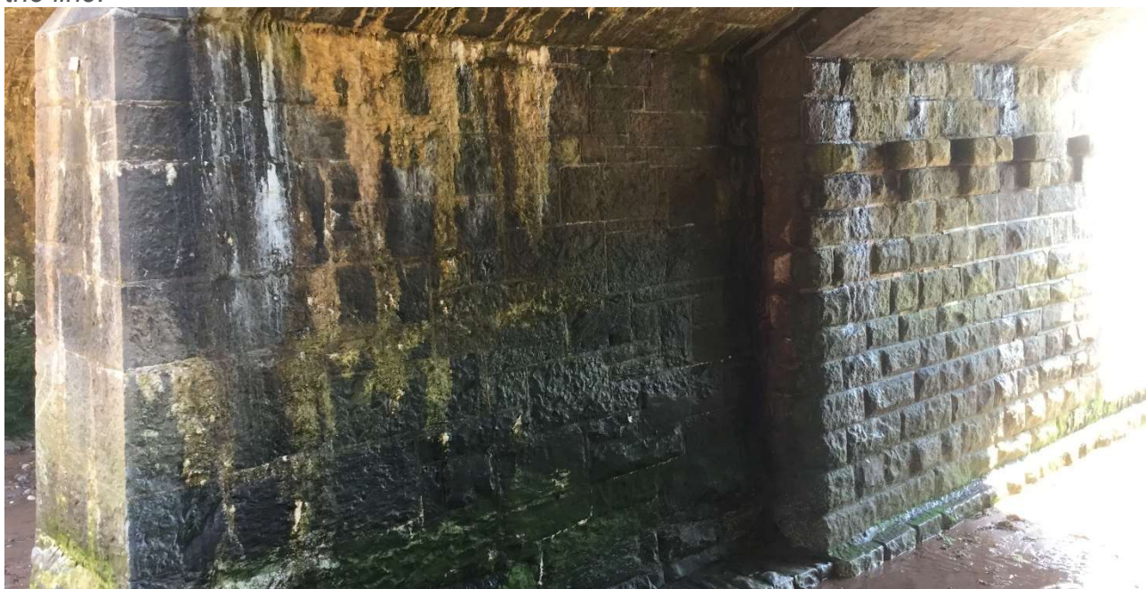
Plate 14 – Showing phasing of the Smugglers’ Lane viaduct due to the doubling of the line.
