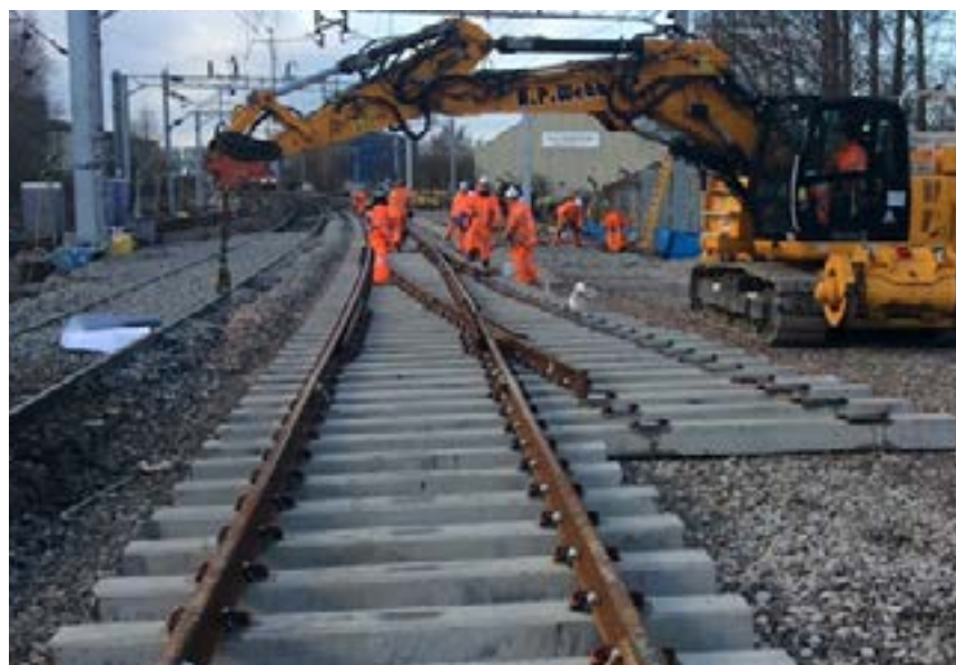
Figure 6: Engineering works to provide new infrastructure at Soho North Junction as part of Birmingham New Street re-signalling
