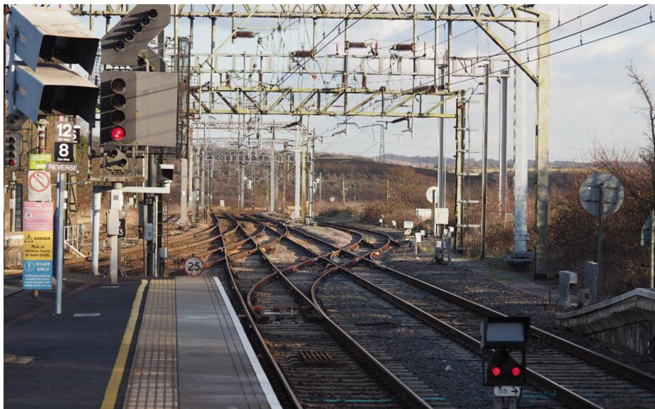
Pitsea Junction, where the Main Line and the eastern end of the Tilbury Loop join.
